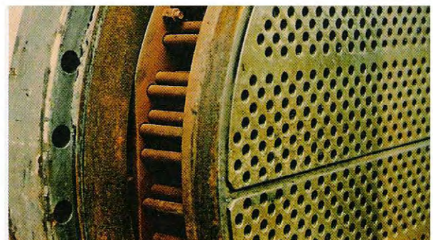
Floating head bundle of a distillation in a crude oil refinery. Tube side and shell side coated, after a service life Of 5 years
